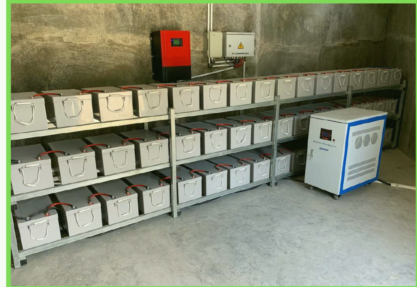
BANK of BATTERIES 48x 200Ah
