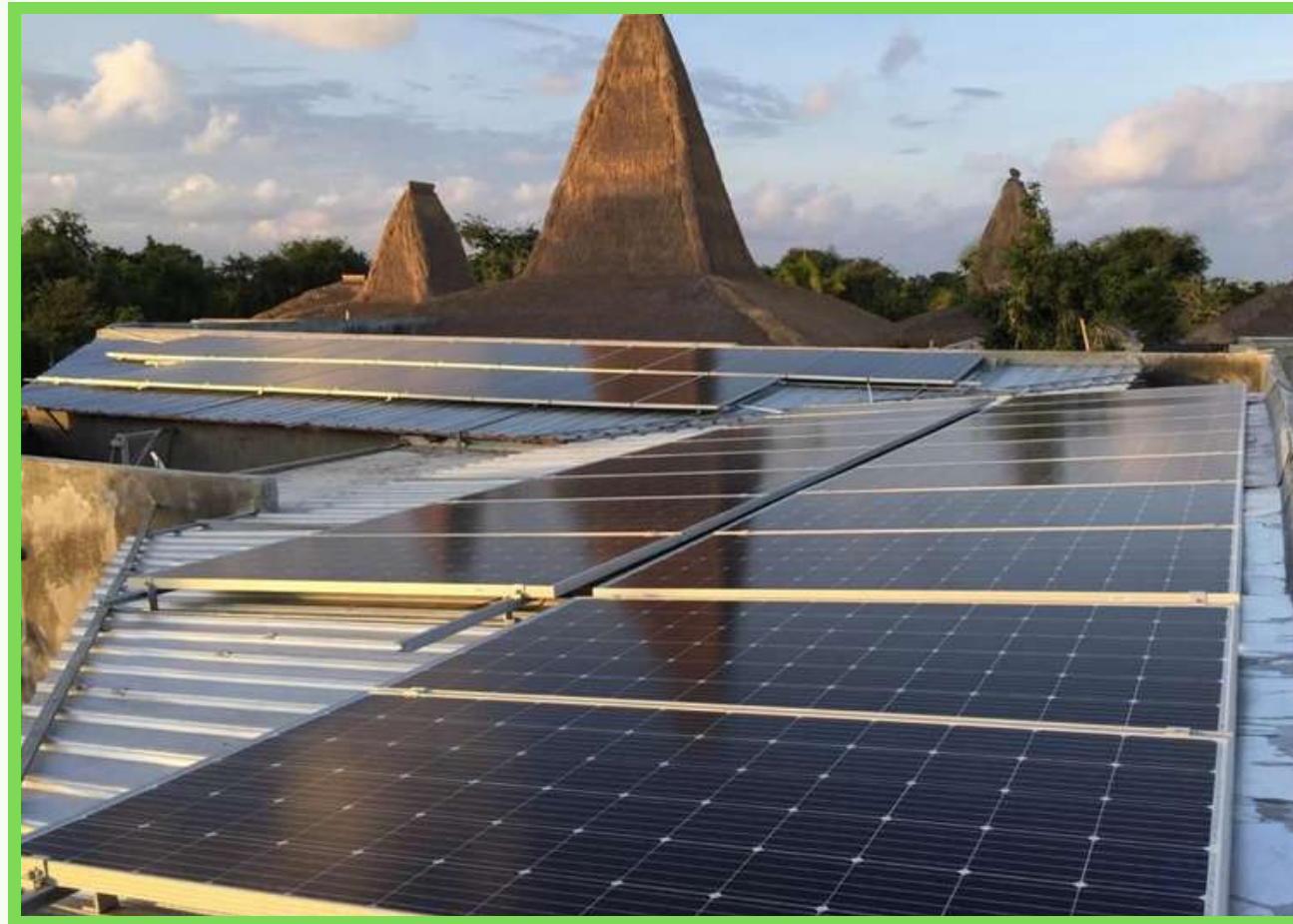
STRINGS OF SOLAR PANELS 20,000Watt
